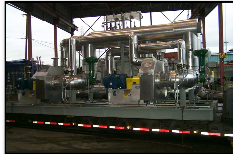
Skids fully commissioned prior to shipping
